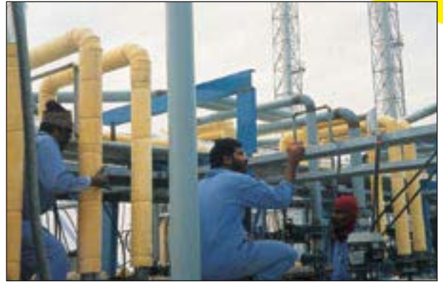
AL KHALEEJ SUGAR REFINERY - JABAL ALI, U.A.E.
